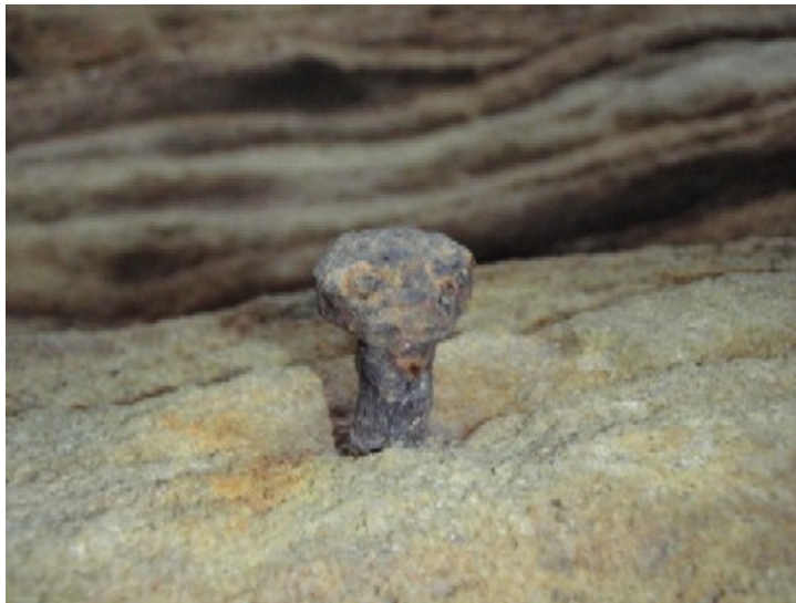
Figure 8 Mildly corroded mild steel bolt on seacliff
