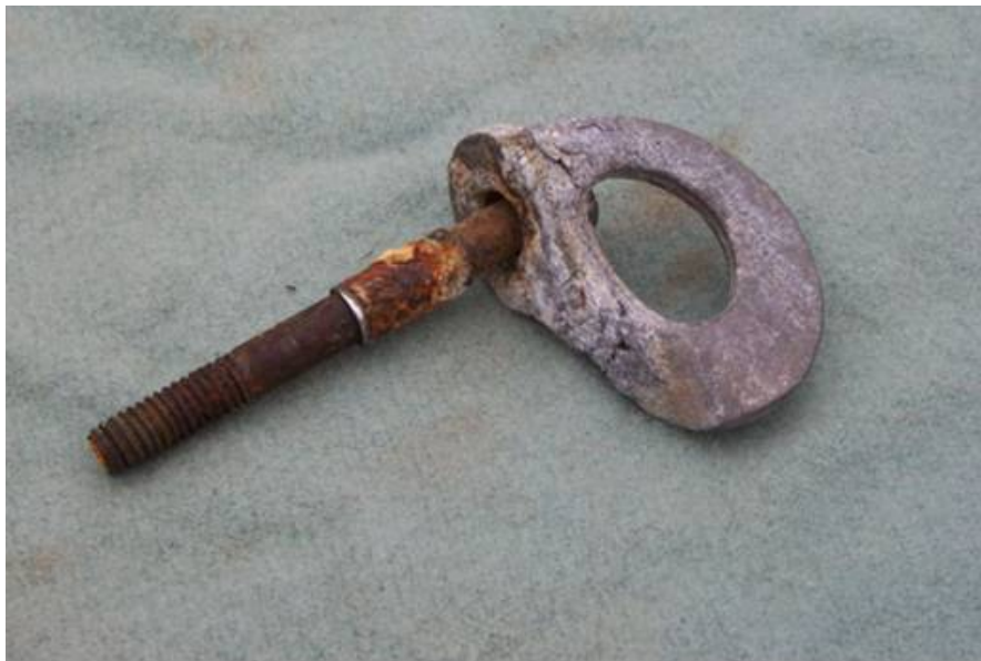
Figure 4.2 Corroded Rawl bolt with evil aluminium hanger. Galvanic corrosion causes rapid corrosion, don't even think of mixing metals.
